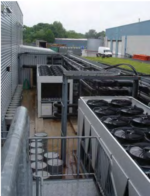
DeltaChill™ FreeCool chillers providing free-cooling to indoor units in a Manchester data centre
